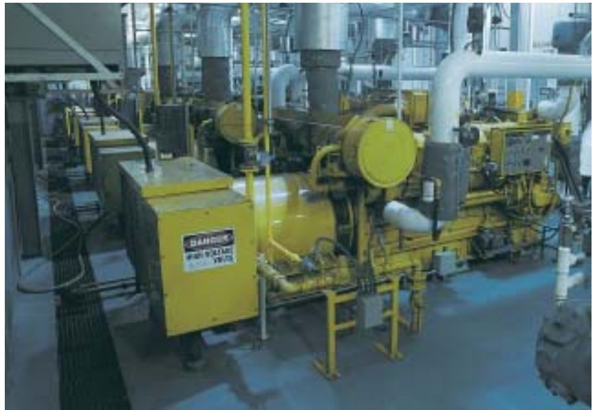
This electroplating company in Ontario uses a natural-gas fueled cogeneration system to supply hot water for the electroplating process.
